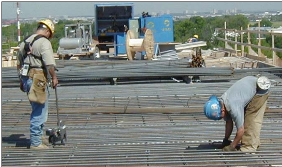
Figure 1: Rebar tying using a rebar tying machine (left) and manual tying using pliers (right).
